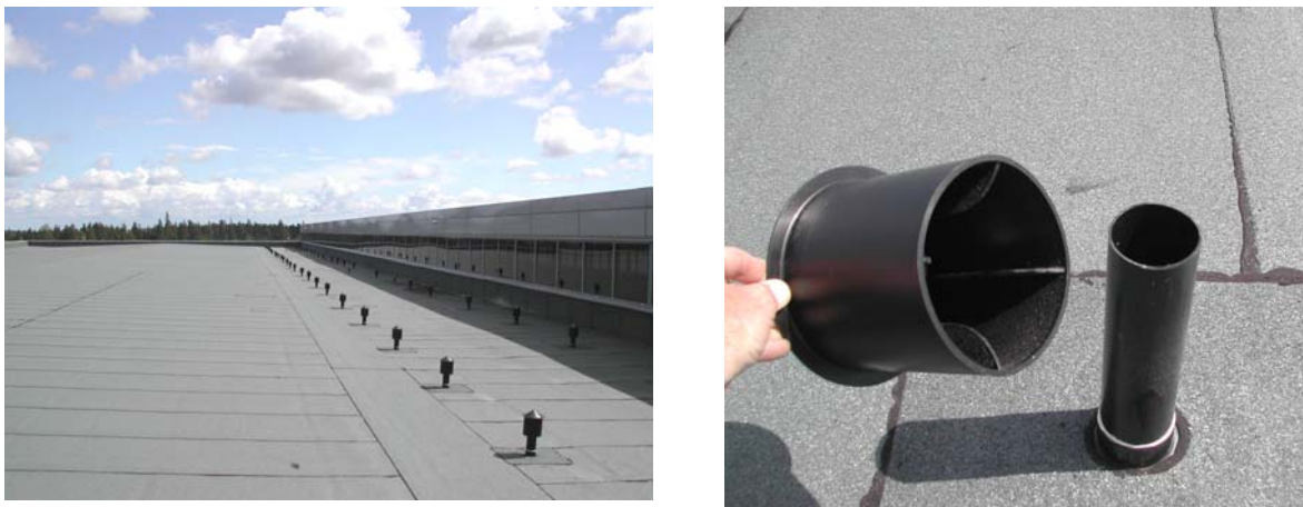
Fig 4. Overview of roof No. 6 in the investigation and details of ventilation louvre (photo: NBI)
