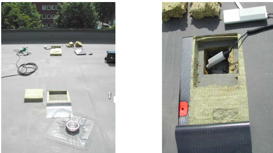
FIG. 1: Roof No. 11. A building from 1980 that was re-roofed late autumn 2000. Pictures taken during survey in Phase 1 June 2002.
